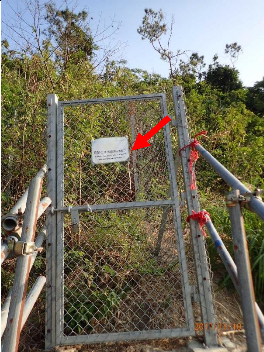
Photo 2 – Current situation of fencing and warning sign
